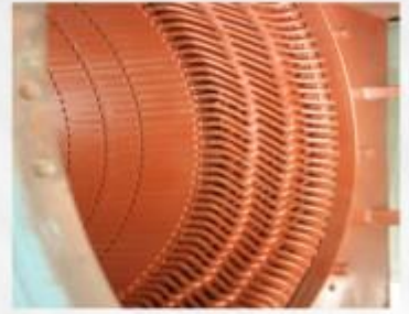
12MW, 6.6KV, 8P STATOR REWIND
