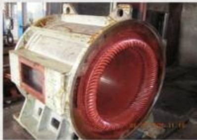
1500KW, 415V STATOR REWIND
