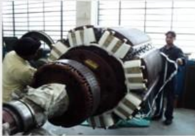
8 MVA, 8 P SYNCH ROTOR REWIND
